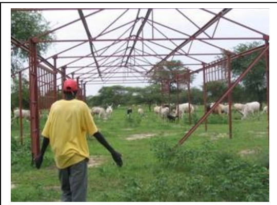
Steel frame for the new Yomchiir Primary School. Permanent cement walls are planned in December 2005. $20,000 is needed by December to construct the school
